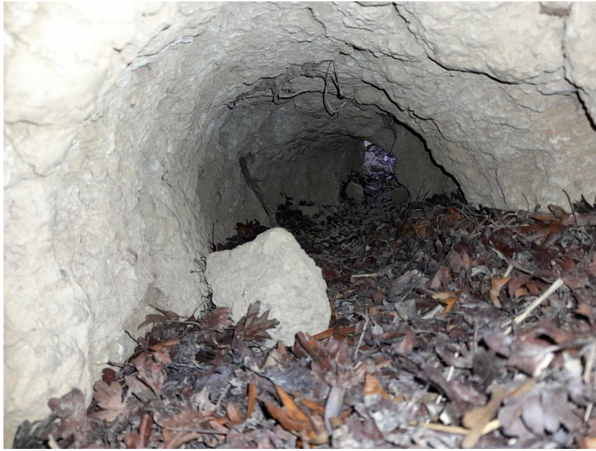
Photo 11. A typical view inside the S6 tunnel, taken through the collapsed tunnel
