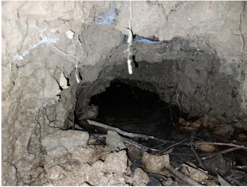
Photo 9. S5 entrance which was flooded at the time of the survey
