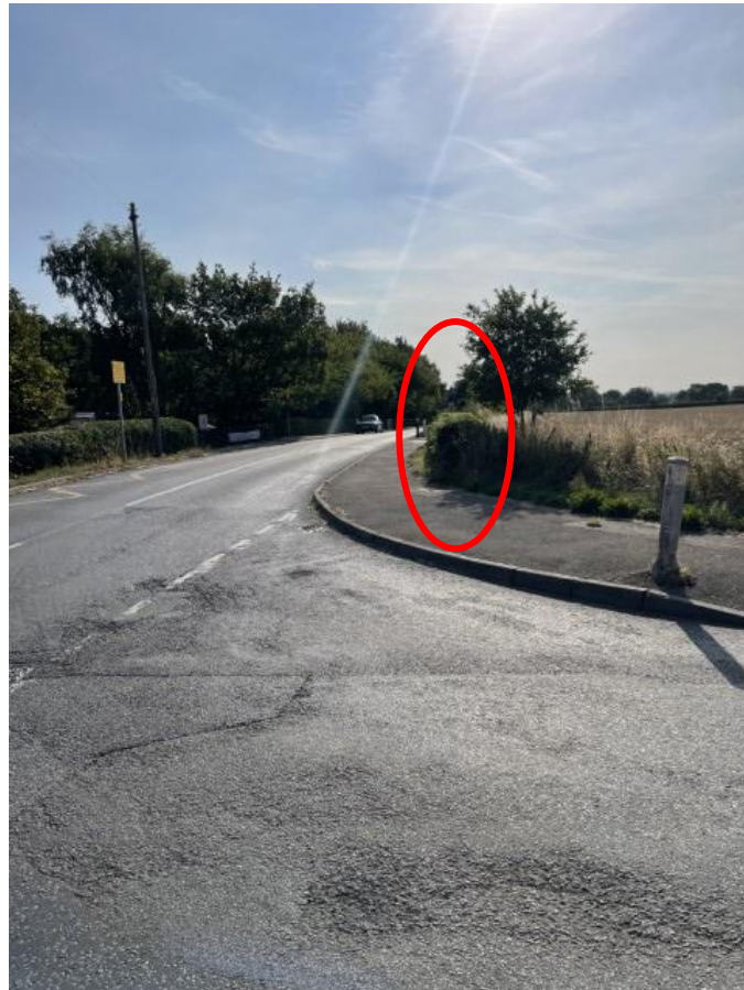
Visibility splay restricted to the right at Foxton Road
