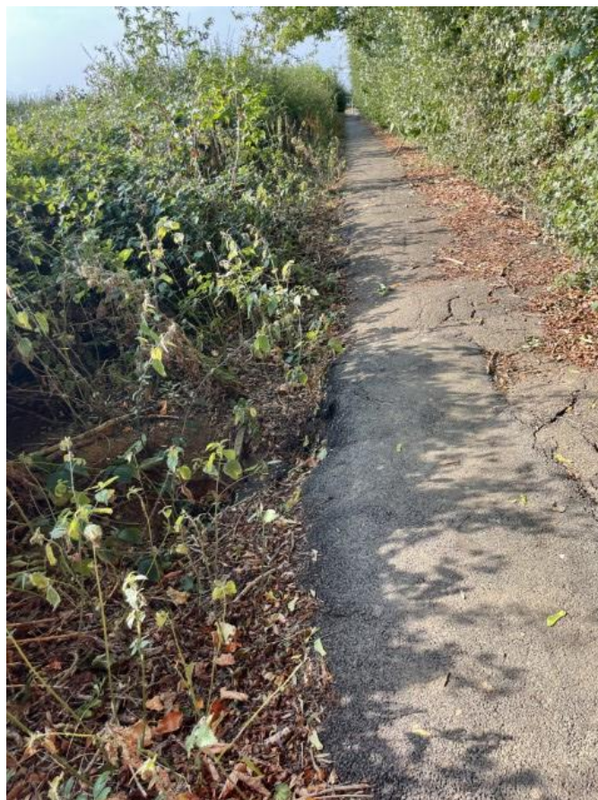
Footpath with steep gradient and drop offs at the edges
