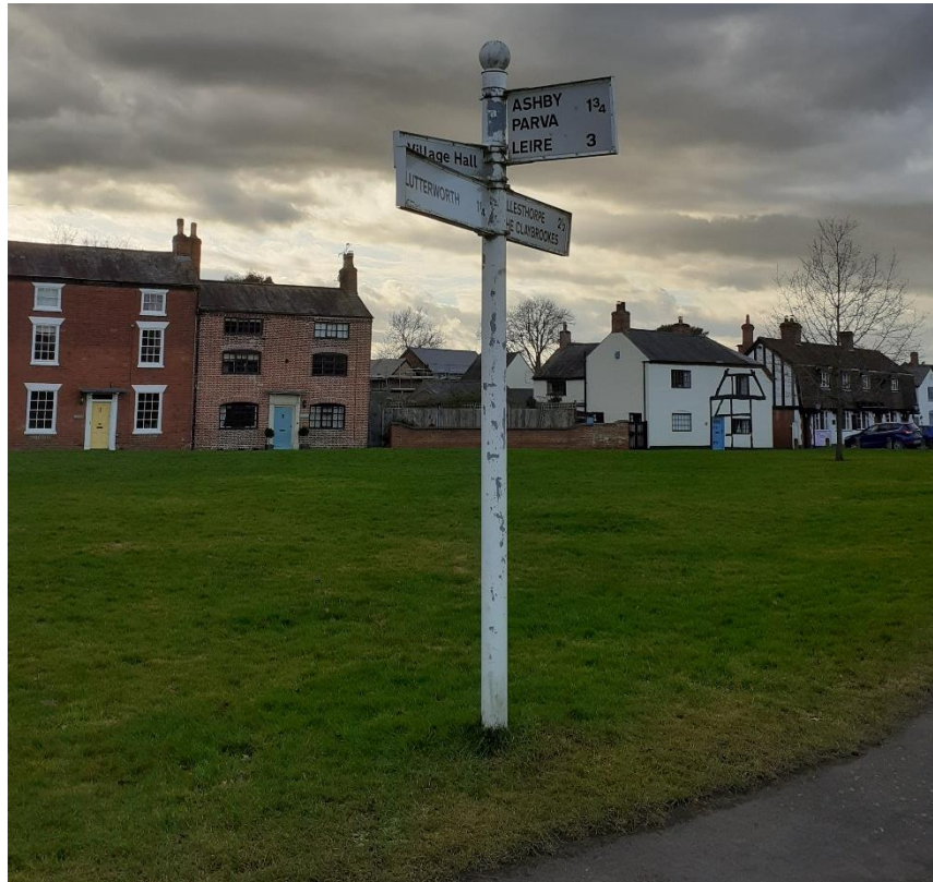
Image showing peeling paint on fingerpost
