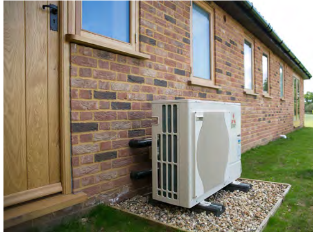
Figure 46: Air source heat pump unit located to the rear / side elevation of a dwelling, so to avoid its visual impact on the dwellings frontage and wider streetscape.
