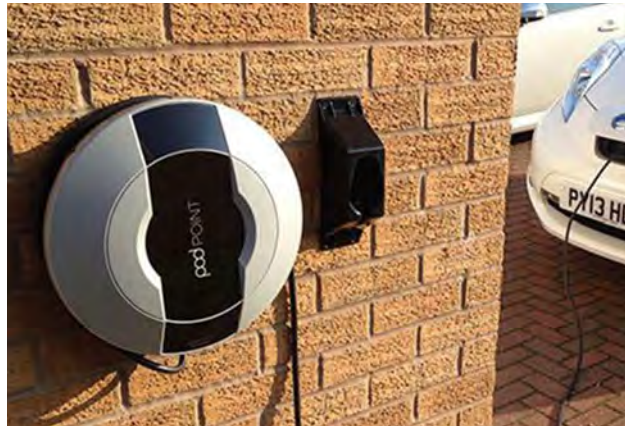
Figure 49: Home electric vehicles charging point
