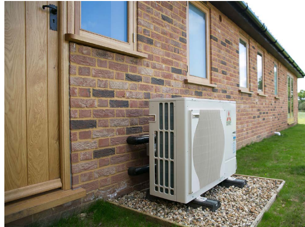
Figure 50: Air source heat pump unit located to the rear / side elevation of a dwelling, so to avoid its visual impact on the dwellings frontage and wider streetscape
